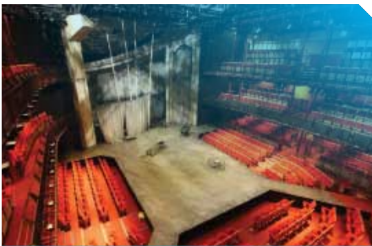
Ampetronic hearing loop installed in Royal Shakespeare Courtyard Theatre, Stratford upon Avon, UK
